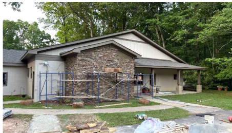
Daniel Hall Daniel hall got a new roof, new paint, and a rock front that will feature a raised, backlit, cross when completed. This rock look and paint colors match the other buildings and sign at the camp.
