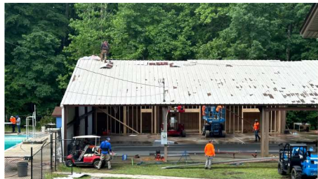
Pavilion Work is finishing up on a new roof over the pavilion with rooms along the back for storage and pool equipment usage.
